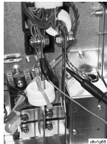
Test points for the secondary voltage from TM1
